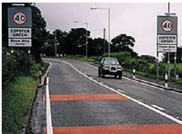
Repeated red patches and speed limit signs, Dorrington
