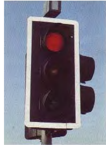
Backing board fitted to increase conspicuity.
