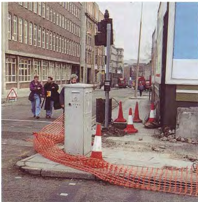
Inadequate provisions made for pedestrians during works
