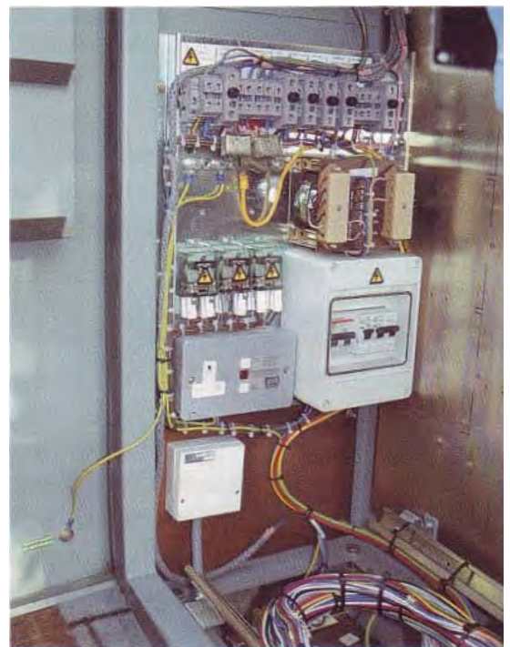
A typical traffic controller installation.
