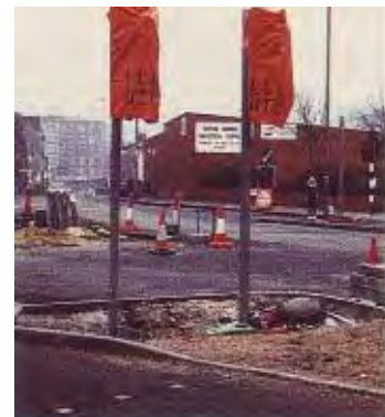
Signals bagged over when not in use.
